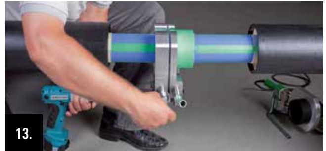
After the cooling time release the clamping jaws on the pipe side by unscrewing the fixing screw.
