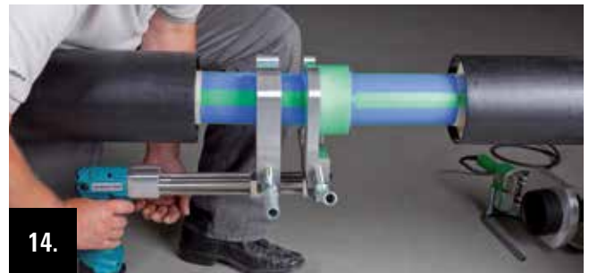
Drive the welding jig apart to release the fixing screw of the fitting clamping jaw.
