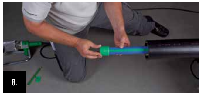
Align and momentarily fix the welding socket. Further processing is carried out after the specified cooling time.
