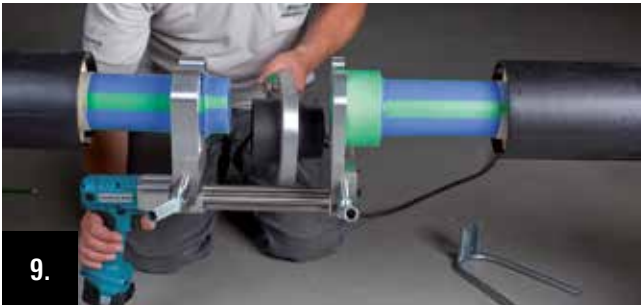
After the end of the heating period drive the welding jig apart and remove the welding device between pipe end and fitting.
